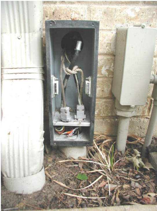
Figure 21. Feed-line entry ground. The PVC pull-box protects the connectors. The aluminum plate grounds the coax shields to the ground rod shown in Figure 10b.
