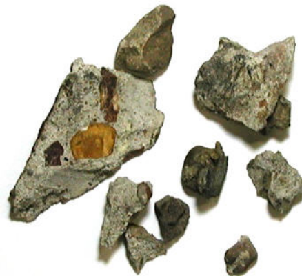
Figure 23. Concrete fragments from footer of foundation. Slab was undamaged, but the over-pour had these fragments blown off - from near the ground rod in Figure 10b.
