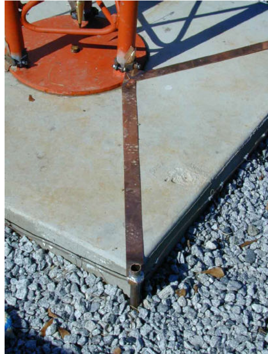
Figure 11. W8JI tower ground. Note the copper straps to pad corner ground rods and copper wire bonding the rods together. See www.w8ji.com for this and other practical installation guidelines.
